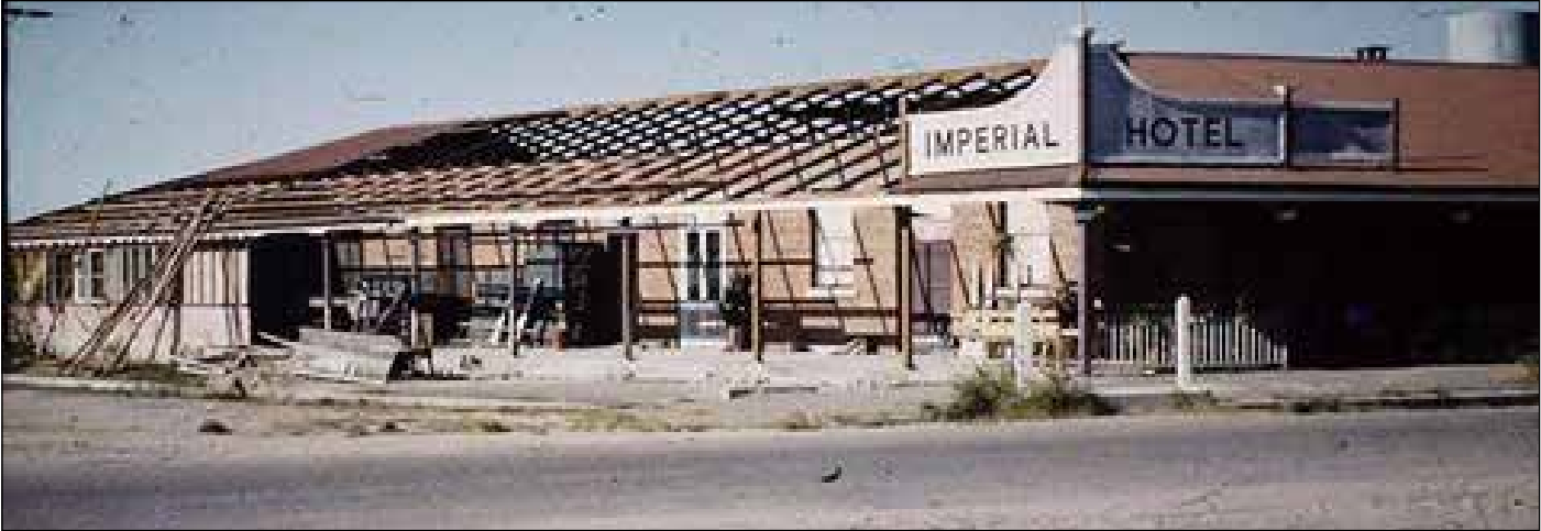
Imperial Hotel, Brandon - damaged after a cyclone
