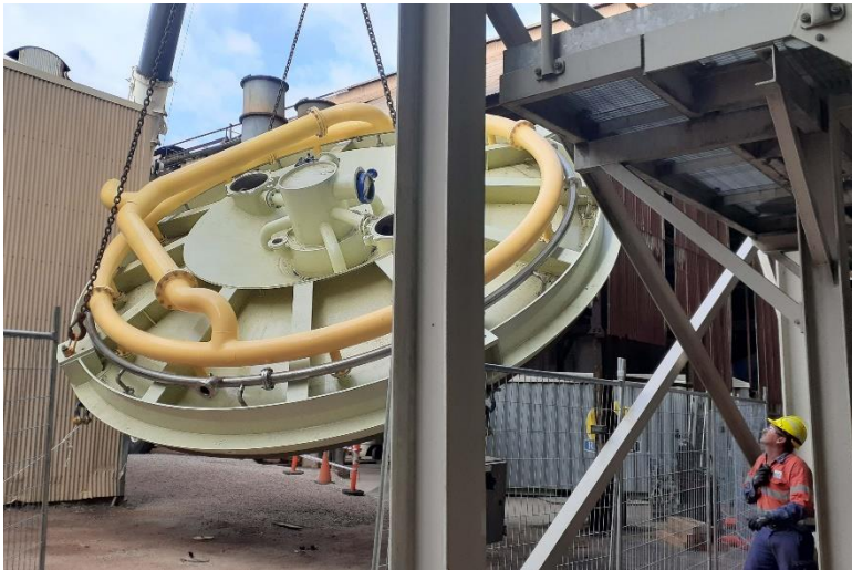
Rigger Pete Daley directs the flip for the bottom cone of the new evaporator at Kalamia Mill.
