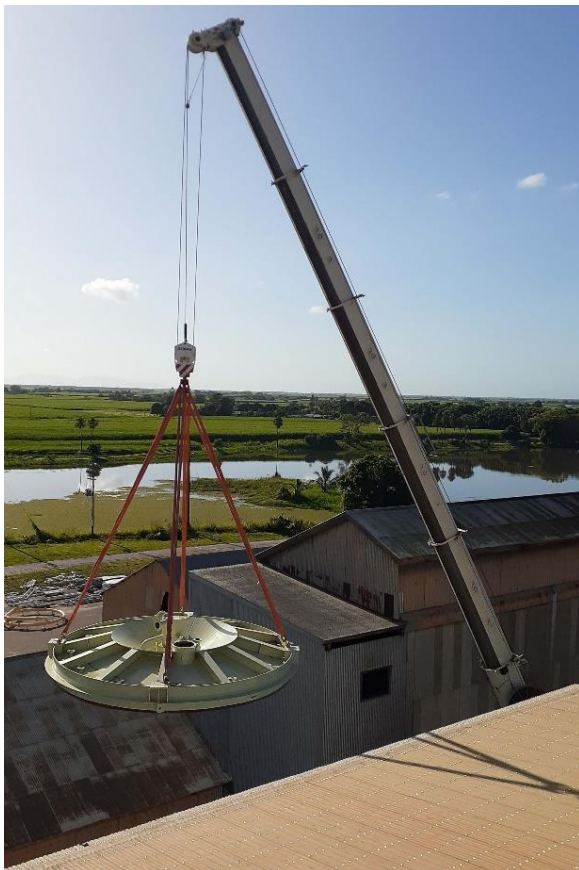
A crane is used to lift the bottom cone section of the new Kalamia Mill evaporator into the factory.
