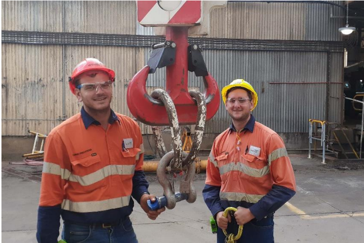
Wilmar Sugar boilermakers Chris Previtera and Joel Hanson de-rigging the crane hook after flipping the bottom cone of the new evaporator on Tuesday (February 15).
