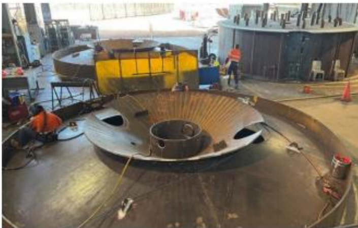
Project work is on track for the two evaporators being built in-house at Wilmar Sugar's workshops ahead of the 2023 season.
