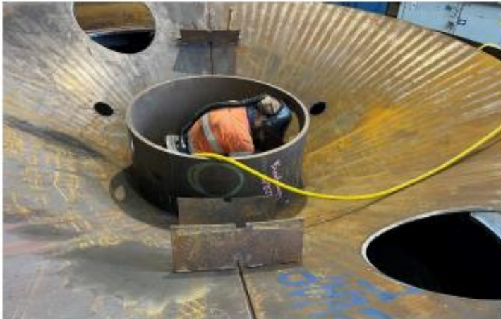
A Wilmar boilermaker works on one the evaporators being fabricated at the Burdekin Centralised workshop.
