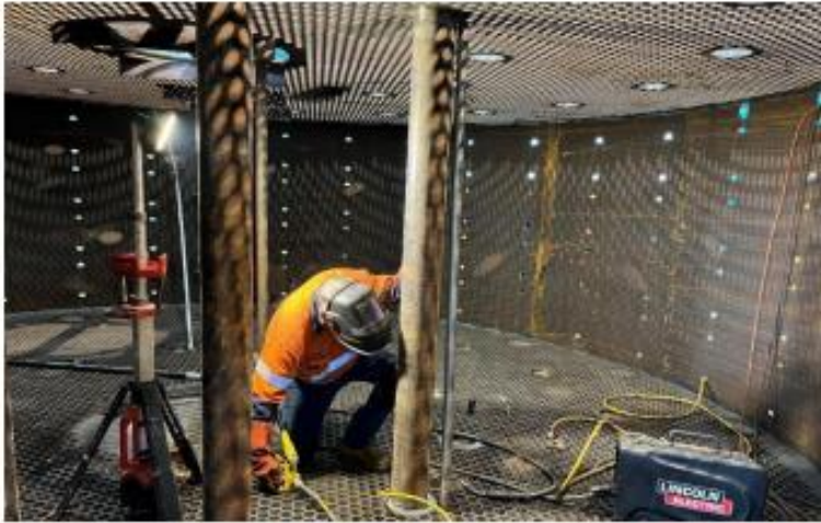
A Wilmar boilermaker welds pipes into the calandria of one of the new Kalamia evaporators.
